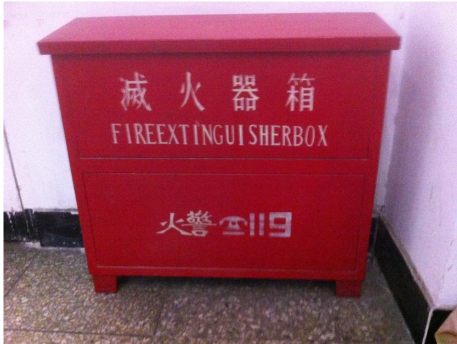
Figure 1c: Fire extinguisher box
