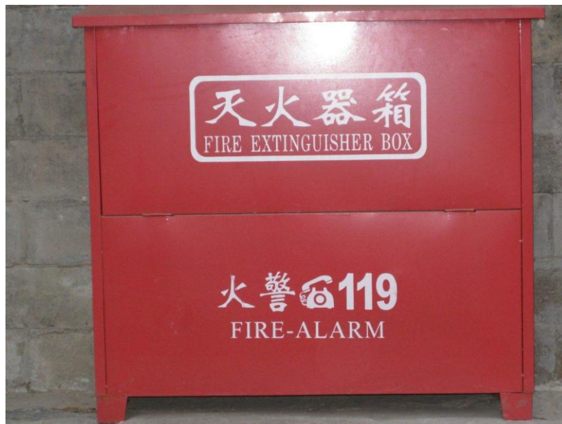
Figures 1a and 1b: Fire extinguisher box
